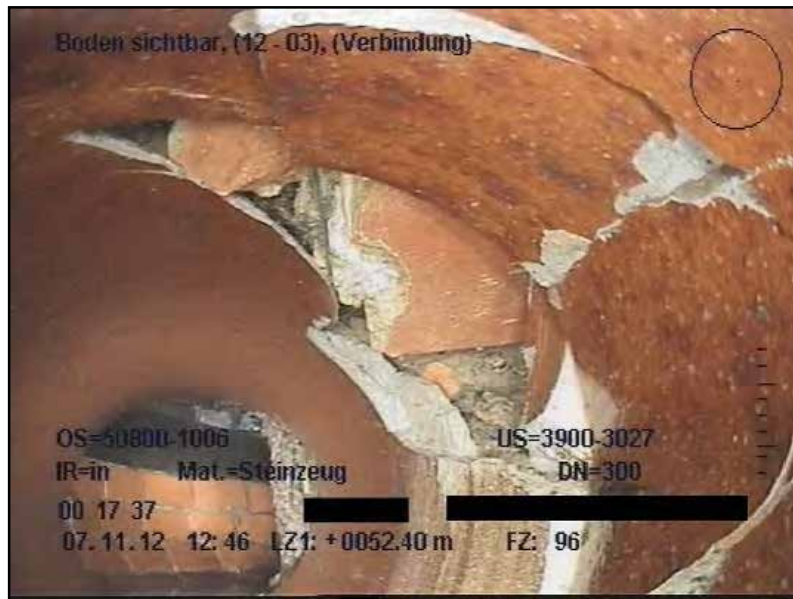
Baulicher Mangel [Rendsburg, 2014]
