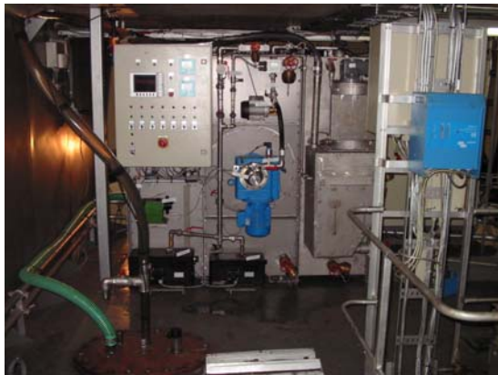
Pilotanlage Martin Systems Engineering GmbH
